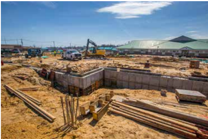
The nearly complete foundation for the $9 million Medical Clinic and instruction building to replace a World War II era clinic at the National Guard Training Center at Sea Girt April 3, 2017. (NJDMAVA photo by Mark C. Olsen/Released)
