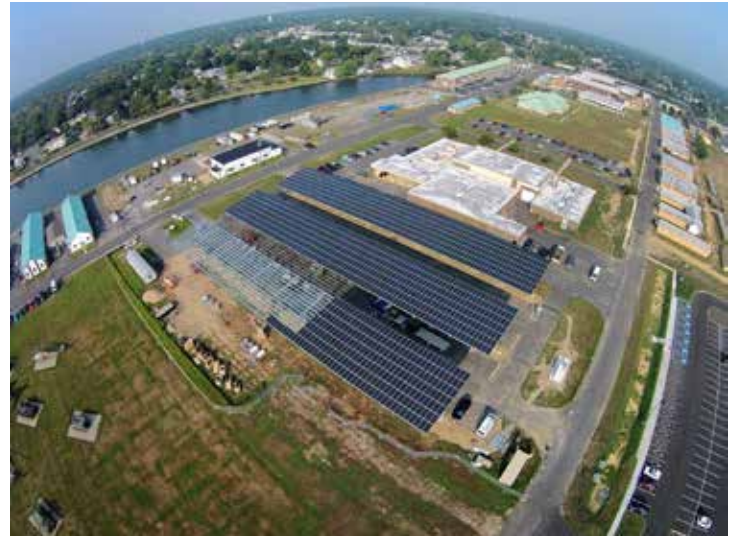
Aerial photo of the photovoltaic project at the National Guard Training Center at Sea Girt, N.J., Sept. 3, 2015. (U.S. Air National Guard photo by Tech. Sgt. Matt Hecht/Released)
